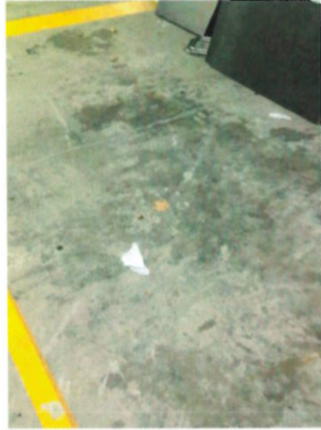
Photo 10: Minor staining with the carpark.
