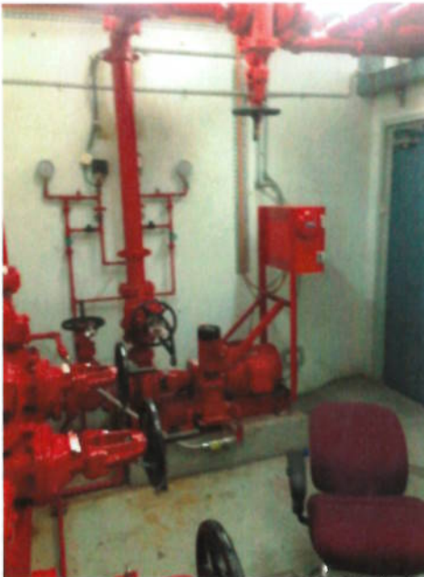
Photo 11: Fire sprinkler system located within the ground level.
